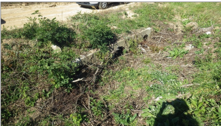
Photo 24 Phase 1 – West Slope at West Sedimentation Pond – Vegetation growth and sediment buildup at inlet of drain structure.
